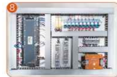
配电箱内部整齐布局 The layout inside the distribution box is in order
